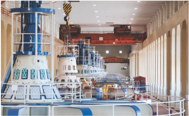
Hydro Electric Power Turbine Generators
