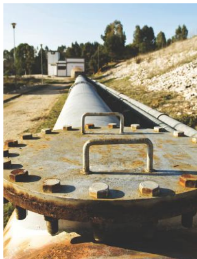
Water Lift Station
