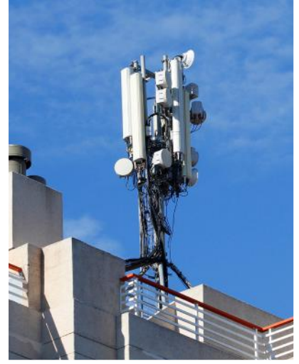
Rooftop Telecommunications Equipment
