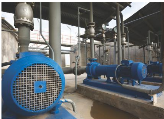
Water Pumping Station
