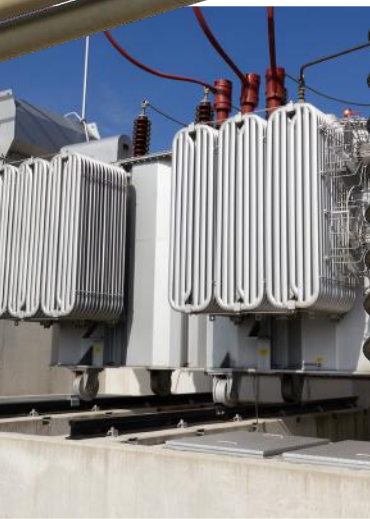
Electrical Power Transformers
