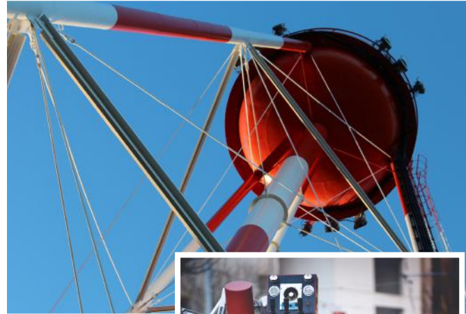
Water Tower with Cellular Radios and Antennas
