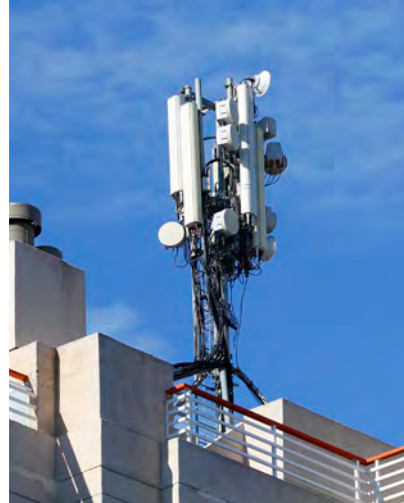
Rooftop Telecommunications Equipment
