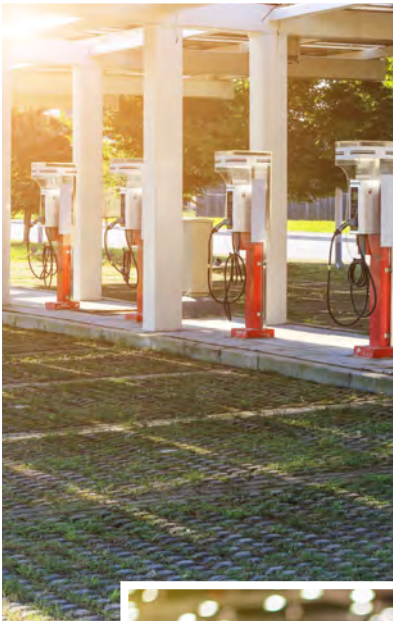
Multiple EV Charging Stations
