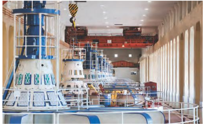
Hydro Electric Power Turbine Generators
