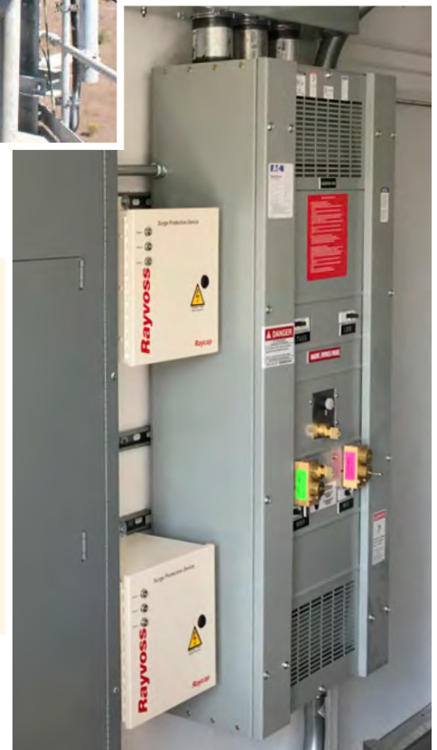
Rayvoss Protecting the UPS on a mobile trailer.
