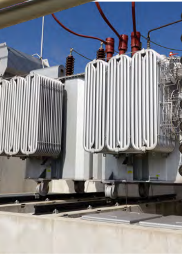
Electrical Power Transformers
