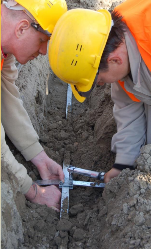
Flat conductor – installation with cross connector
